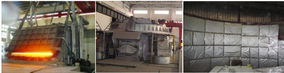
Application on melting and holding furnace
